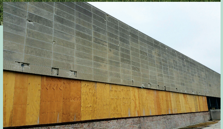
JAHN M70 is being used on the West Elevation of the South Side Water Purification Plant. The mortar was chosen for its ability to replicate the building's "Shot-Shaw" texture and for structural compatibility
